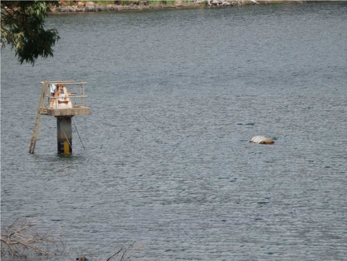
Photo 15: Trunnion for water supply outlet
