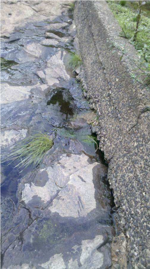
Photo 19: Seepage weir wall with under-seepage (photo taken by Council staff in June 2014)
