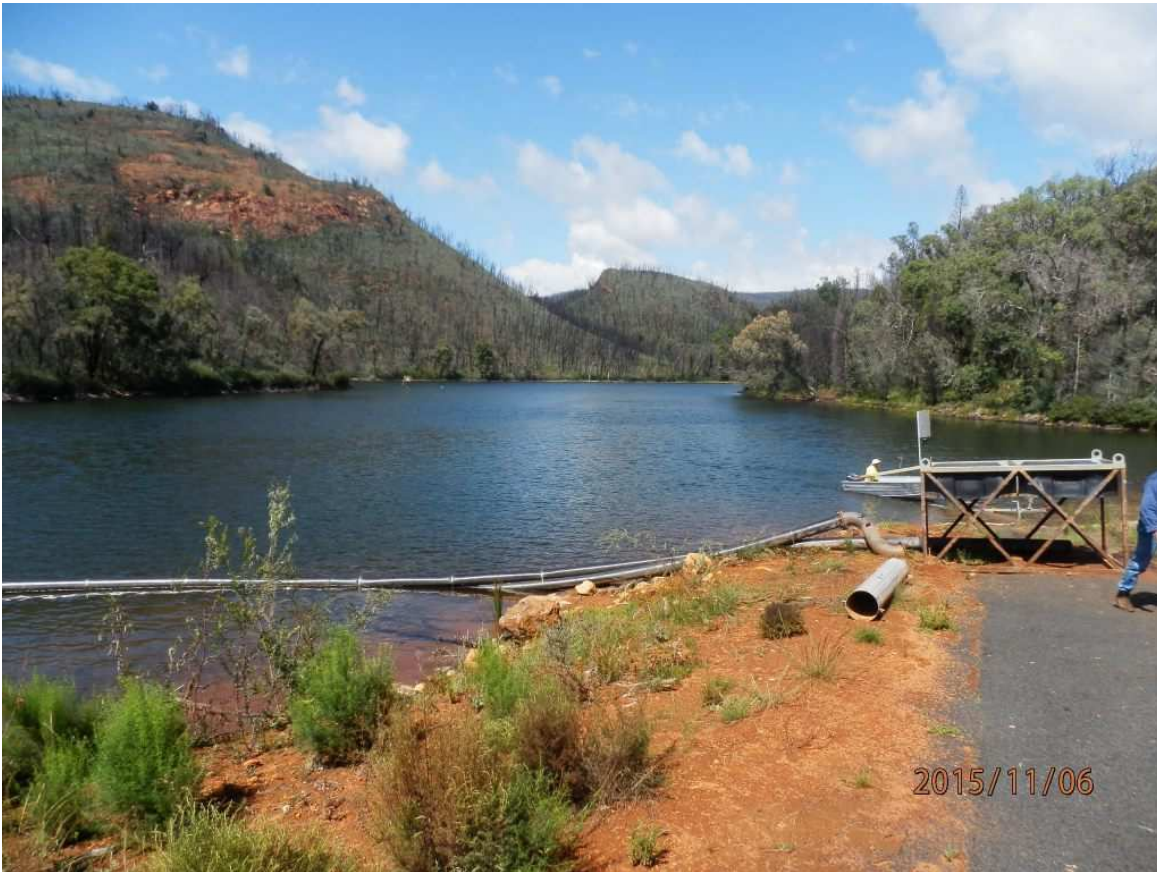
Photo 17: Dead storage line (pump removed for repairs)
